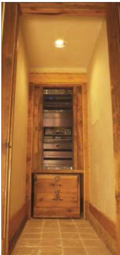
The main equipment location is under the stairs.
